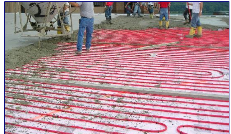
Medivac landing pad on hospital rooftop
