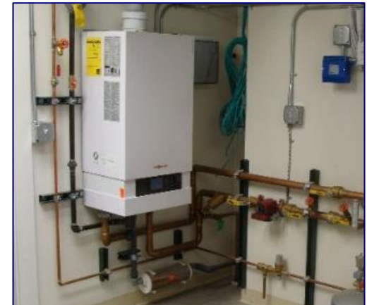
This system will use a dedicated boiler
